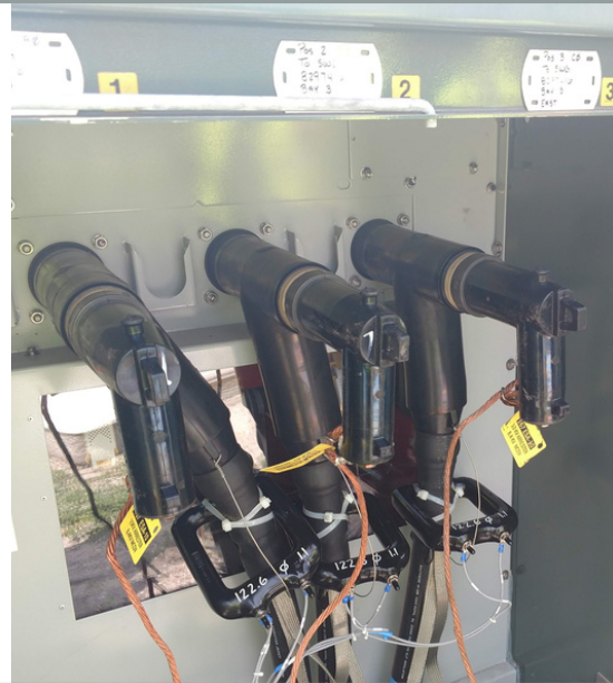
Real time monitoring capabilities of customer installed CT & PT devices.
